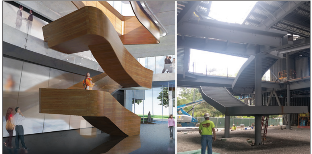
Rendering of the Center for Missouri Studies lobby by Gould Evans architects, left, and the staircase under construction.
