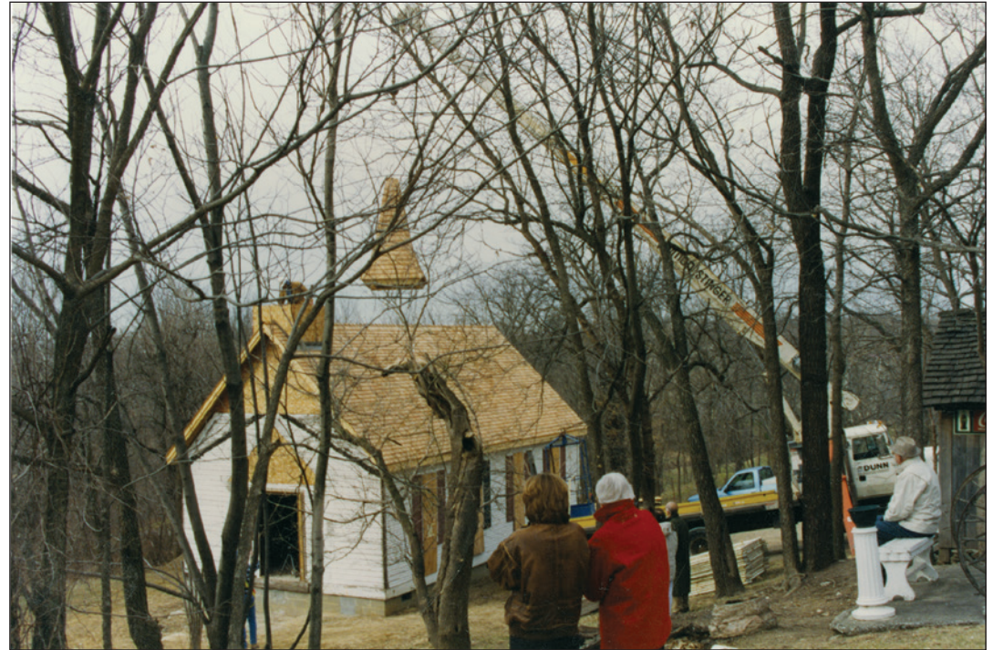
Onlookers watch as a crane places the steeple on top of the newly roofed chapel at Stroud's Oak Ridge Manor.
